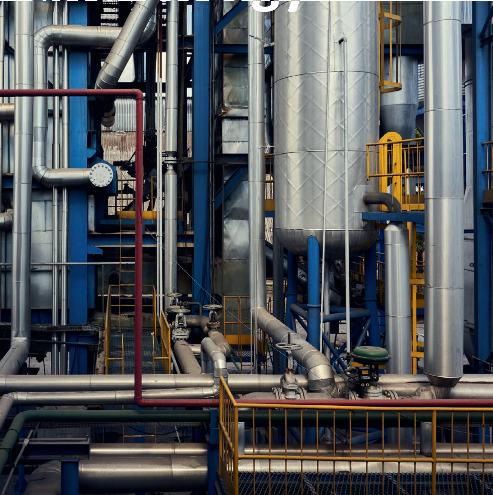
Picture: Biomass power plant, MIL Energia Renovável, Brazil
